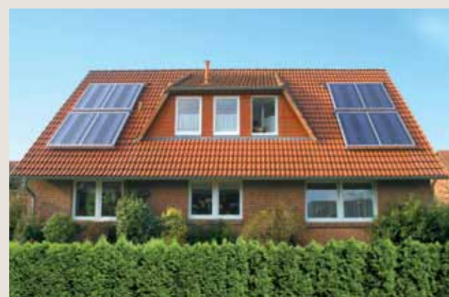
A single-family house in Lüneburg with eight hybrid collectors (20 m 2 collector area) as a rooftop installation. Solar energy yield per annum: 4,050 kWh for heating and water heating, incl. 1,350 kWh of electricity.
