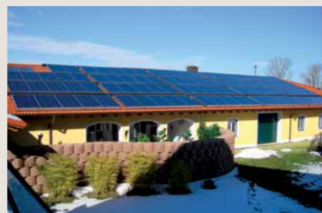
The wellness facility of Hotel Preishof in Kirchham, eastern Bavaria, with 97 hybrid collectors (240 m 2 collector area) as a rooftop installation. Solar energy yield per annum: 67,700 kWh for heating and water heating, incl. 13,000 kWh of electricity.
